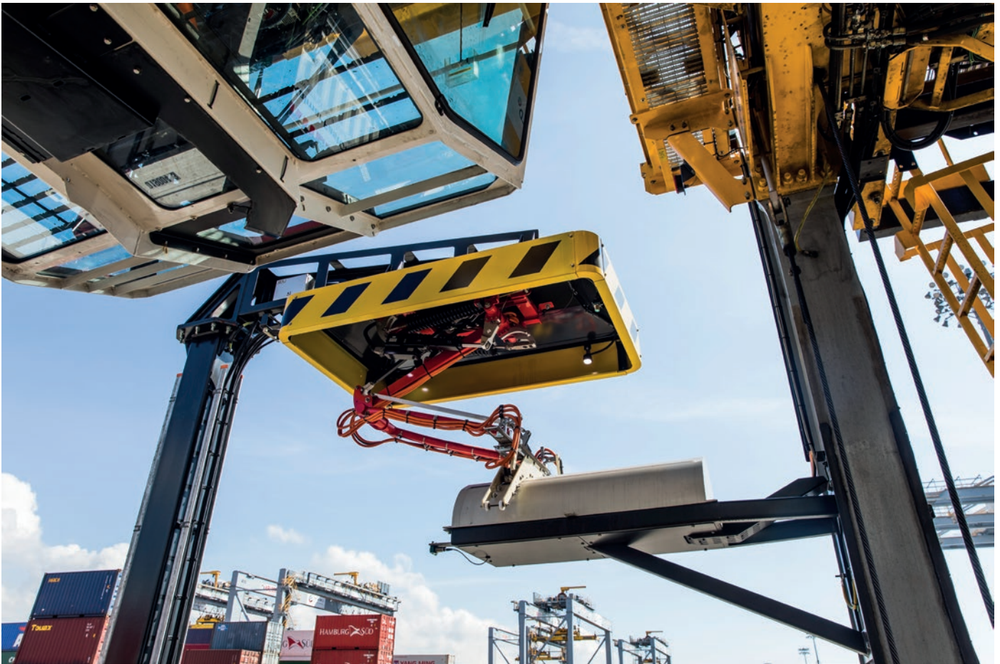
Picture 1. Charging pantograph connected to the machine-side contact dome
